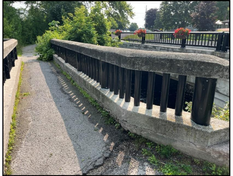
South barrier system
