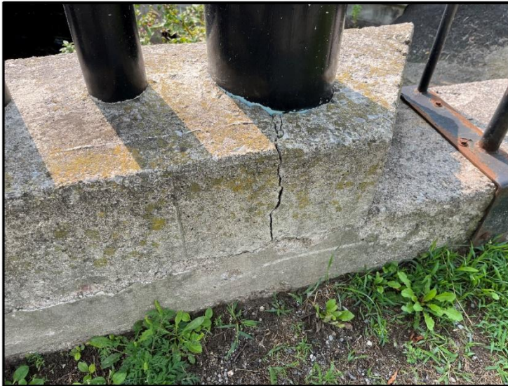
Wide crack in curb
